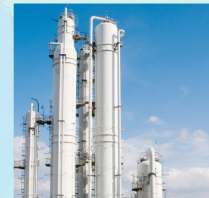
Distillation columns at the JSR chemical plant
